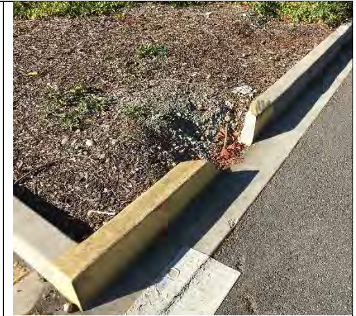
Broken curbing by the southwest parking lot entrance
