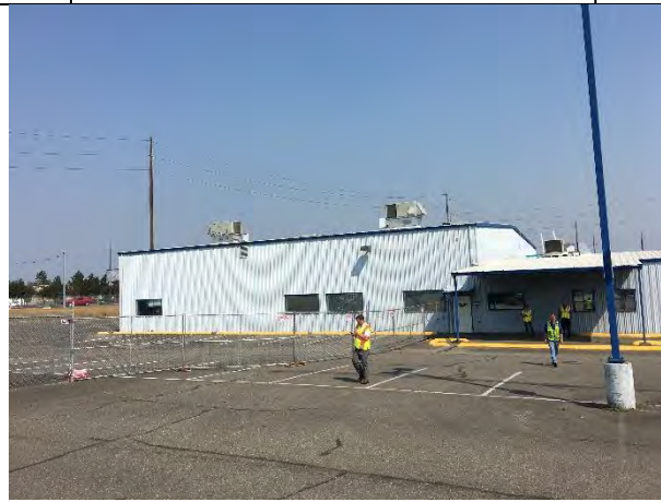
Roof mounted HVAC units
