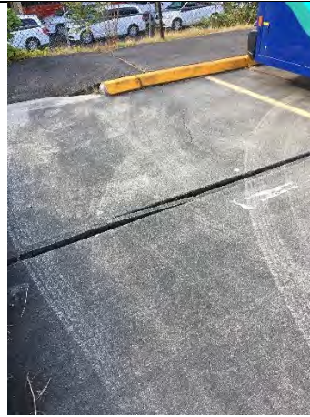
Enlarged concrete joint in southwest corner of parking area
