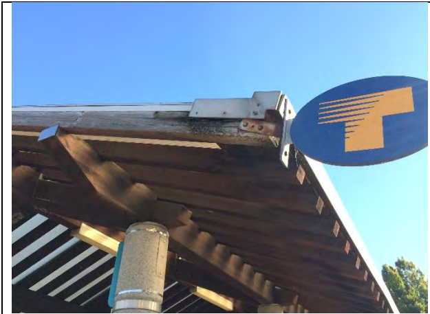
West bus shelter gable rot
