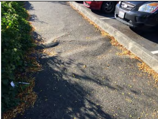
Pedestrian walkway with root growth
