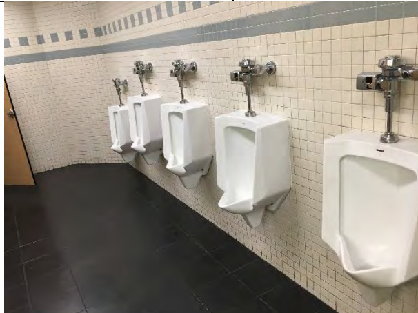
Fixtures in bathrooms are working and in adequate condition
