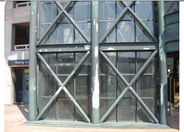
West garage southwest corner elevator tower has peeling paint
