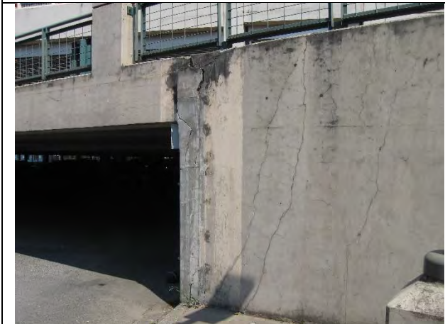
Damaged concrete at ramp on west side of west Garage
