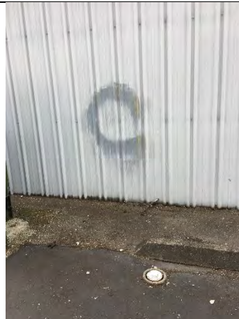
Siding on north wall of building with graffiti
