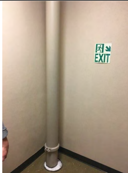
Standpipe in stairway with no hose connections
