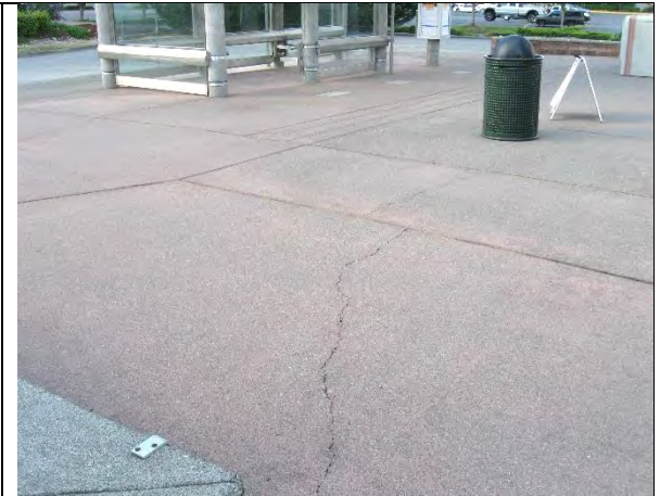
Cracks in concrete walkways
