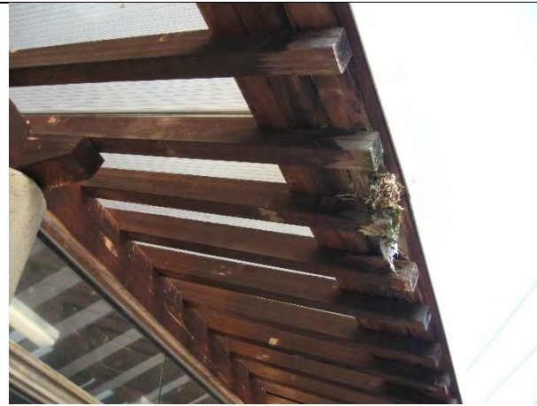
Debris on gable ends causing additional rot
