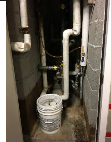
Difficult access for maintenance and repair for the water distribution and sanitary waste for driver break room/rest area
