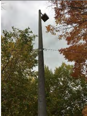
Lighting near utility building
