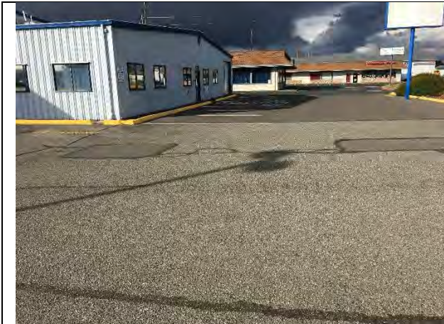
Asphalt cracks have been sealed
