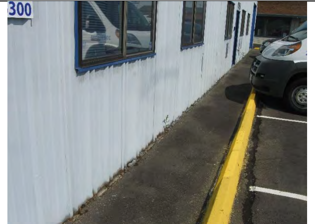
East wall of building, showing rusted siding at bottom edge
