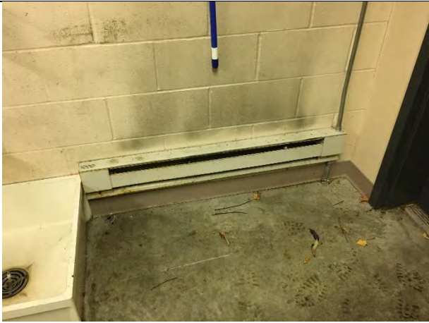
Utility room baseboard heater
