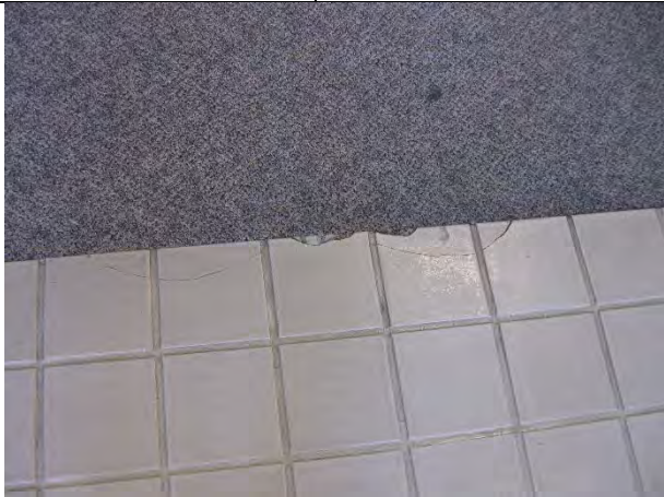
Tile breakage at main entry at door sill and tile to carpet transition
