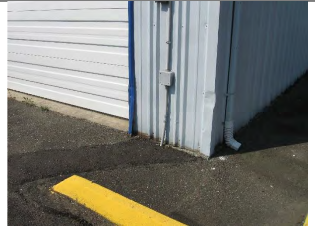
Dents in metal siding and door jamb at roll-up door northeast corner
