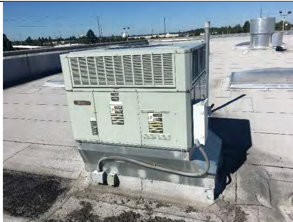
Evidence of low area on roof that collects water and debris from not draining properly
