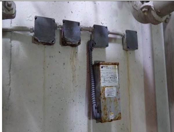
Junction boxes and control transformer in pump room have severe corrosion and should be replaced
