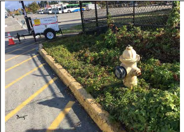
Fire hydrant needs bollards protecting it
