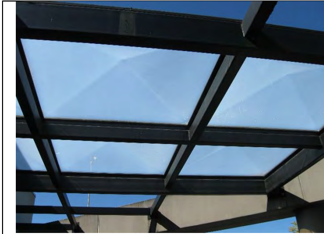
Skylight at entry has dirt in valleys between units
