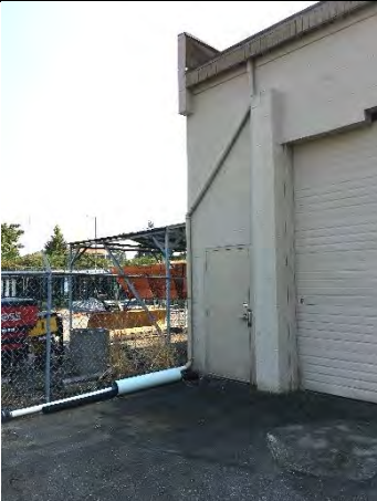
Gutter extended to about 100 feet from building
