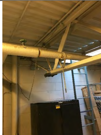
Pipe hanger on second floor is broken
