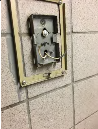
Radiant heater thermostat in public restrooms on the pick-up/drop-off area island
