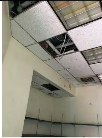
Ceiling tiles missing
