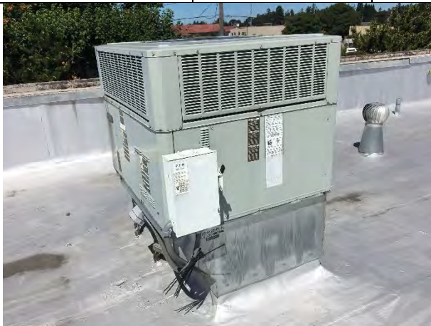
Roof mounted heating and cooling unit
