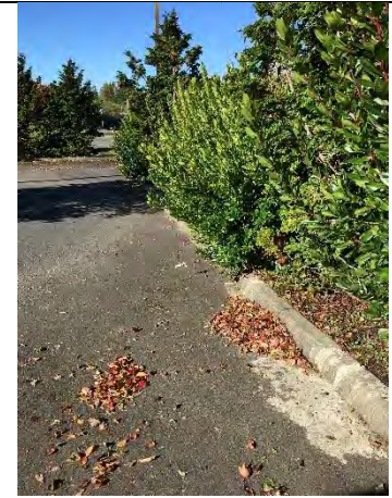
Landscaping needs to be trimmed from parking area
