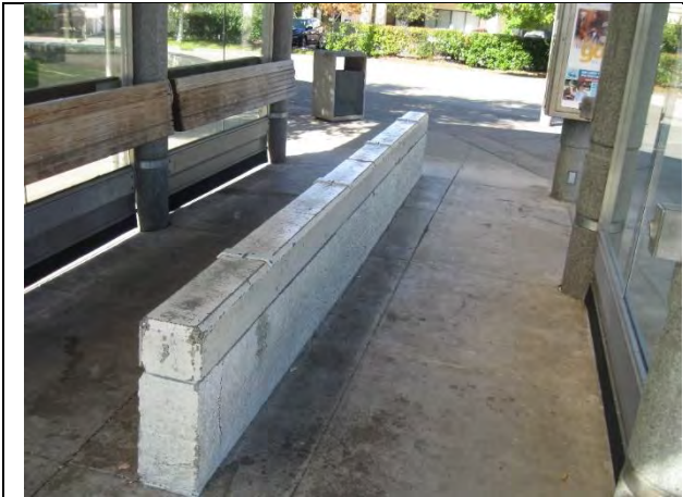
CMU seating in bus shelter – paint is worn
