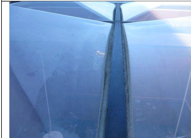
Skylight at operator entry has dirt in valleys between units
