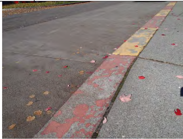
Curb at West side bus pull-up area needs repainting
