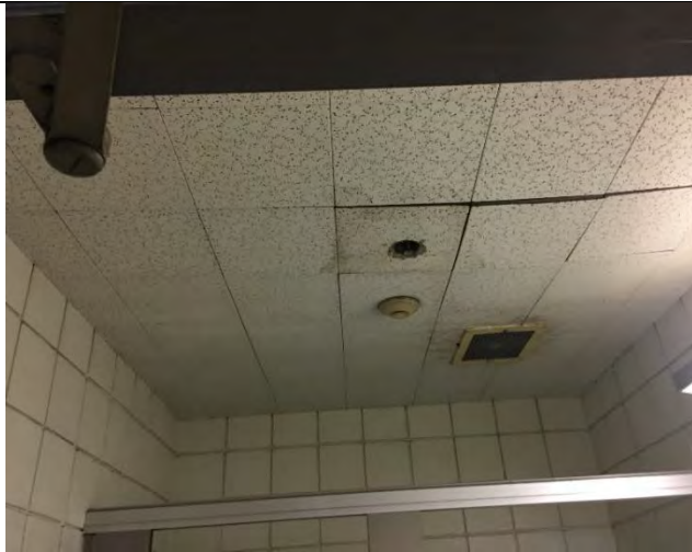
Paint area restroom sprinkler head
