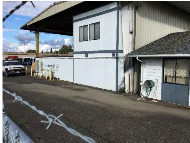
Bollards protecting the electrical panels
