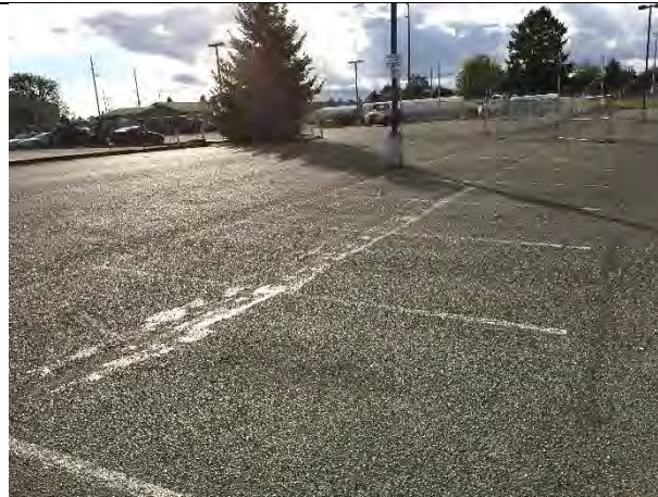
Parking lot striping is faded, but adequate
