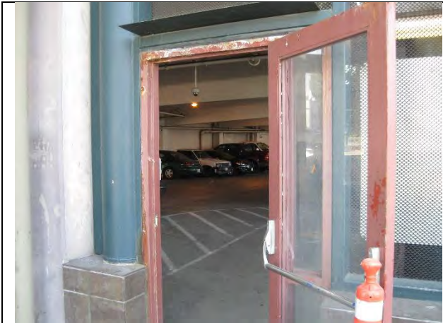
Rusty door frame at northeast corner of east garage
