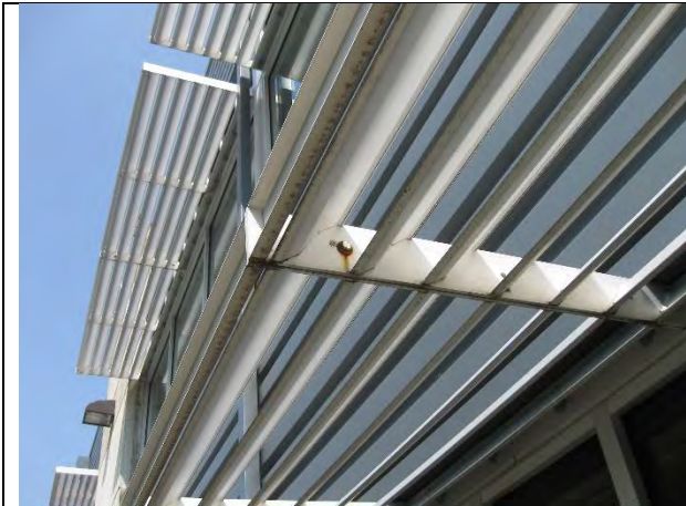
Exterior canopy framing, note rusted bolt/washer
