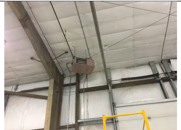
Heater in shop garage
