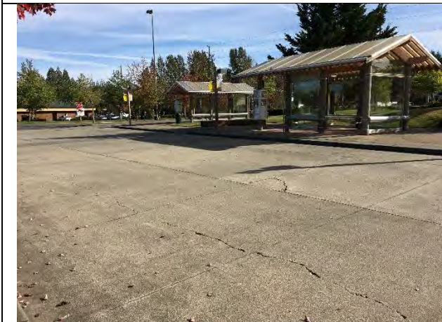
Cracks in interior concrete pavement
