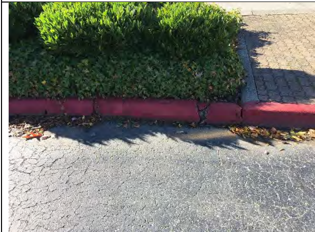
Broken section of curbing
