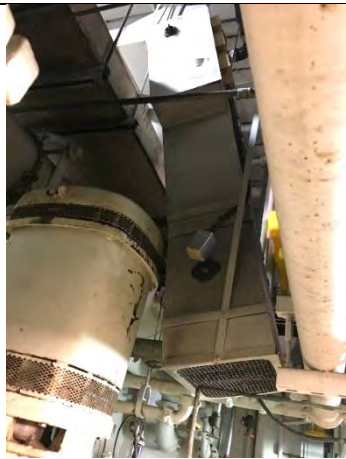
HVAC duct in Pump Room
