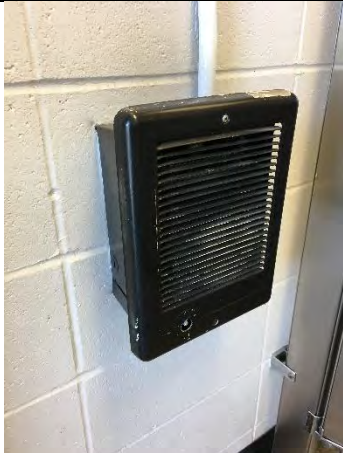
Men's Restroom heater – missing thermostat knobs
