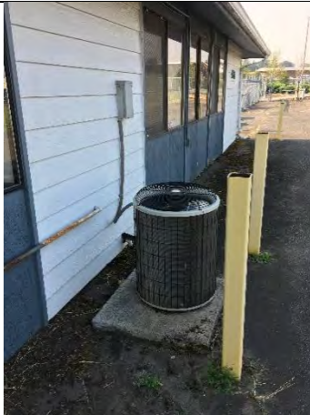
Exterior of HVAC system for service supervisors building
