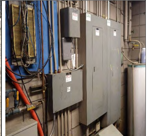
Water heater needs to be seismically restrained
