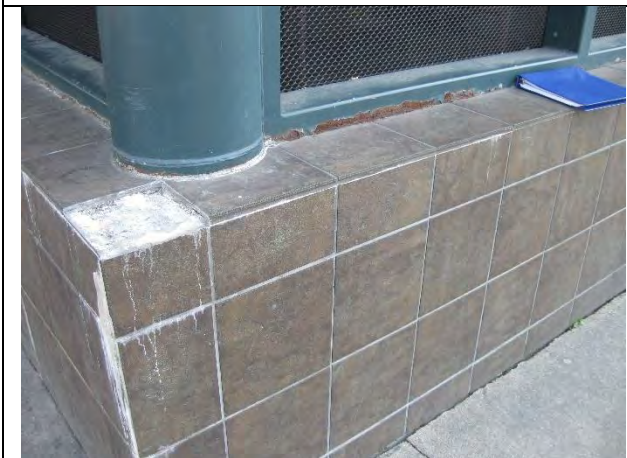
Missing tile and corroded steel frame at northeast corner of east garage
