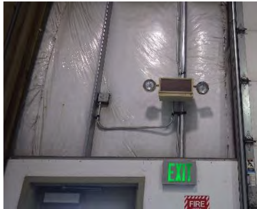
Non-functioning egress light
