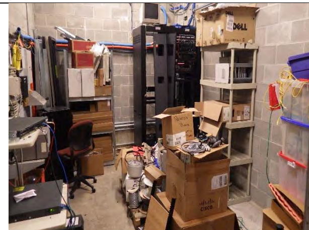
East garage communications room
