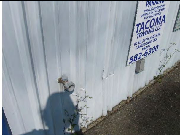
Dents in metal siding at southeast corner
