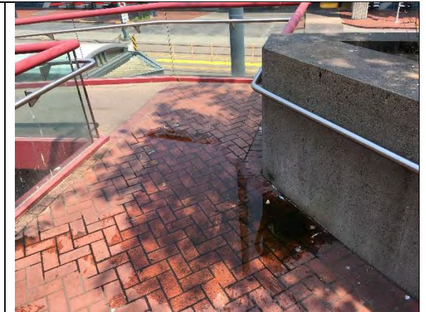
Wheelchair ramp landing with clogged drain
