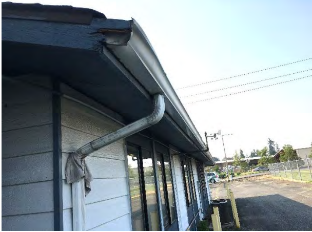
Northwest corner of service supervisors building showing damaged gutter
