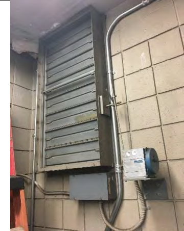
Intake and exhaust louvers located in mechanical room
