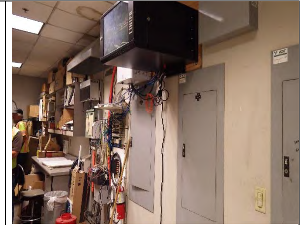
Electrical panel obstruction
