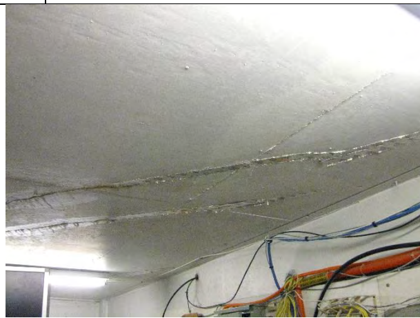
Patched cracks at west garage server room
