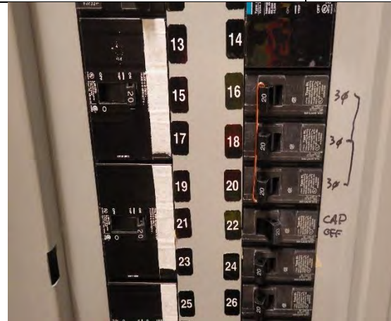
Electrical panel UPS-A located in the second floor server room
