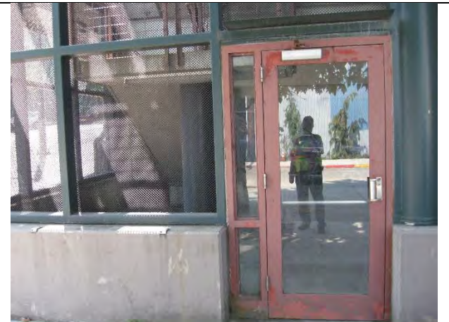
Corroded doorway at southeast corner of east garage
