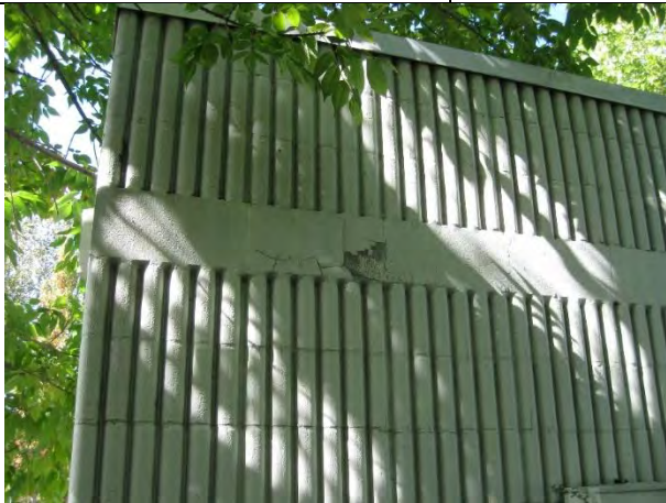
CMU damage on utility building
