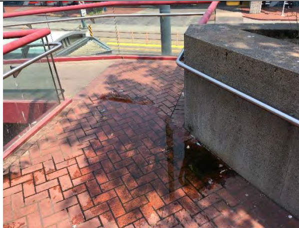
The drain in the walkway at the top of the first wheelchair ramp going up from Commerce Street was clogged at the time of the site visit
