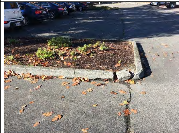
Broken curb and cracked asphalt
