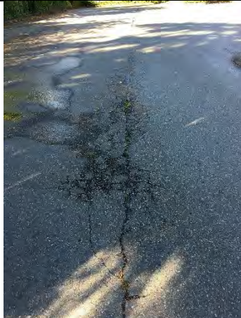
Alligatored asphalt in parking lot
