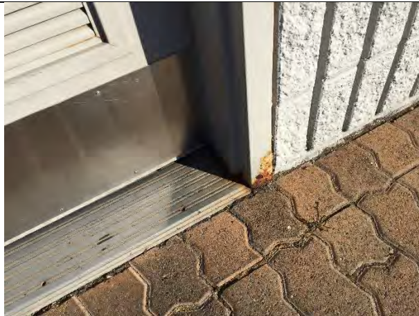
Rust on doors of bathroom at the utility building
