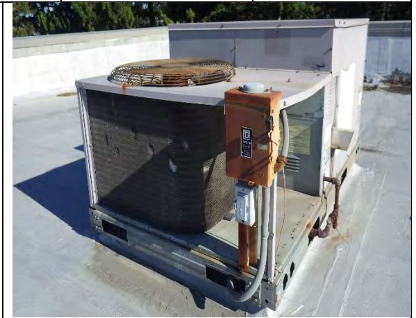
Rooftop electrical disconnect protective coating has exceeded useful life
