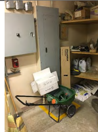
Relocate items located in front of electrical panel
