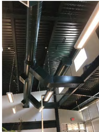
Bus Shop (west end) HVAC distribution system
