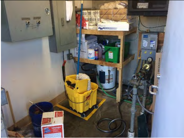
Valves and controls in utility room in utility building
