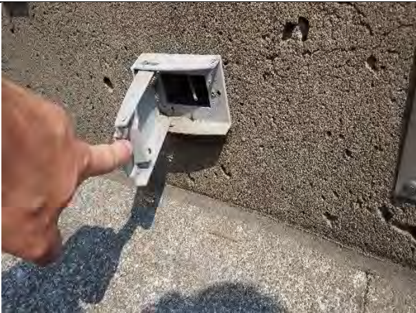
Junction box at north end of plaza have receptacle missing leaving access to exposed conductors
