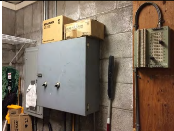
Electrical equipment in utility room
