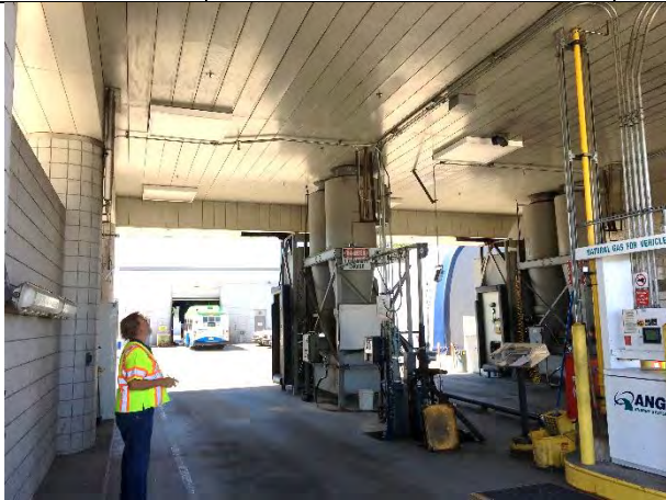
Small air leak in compressed air piping at fuel island #2
