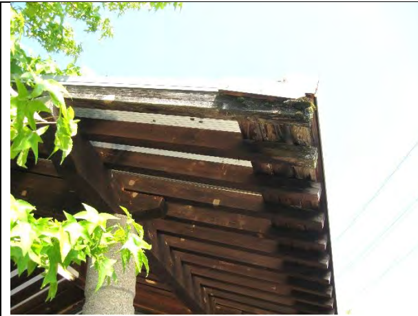
Shelter gable ends are rotting
