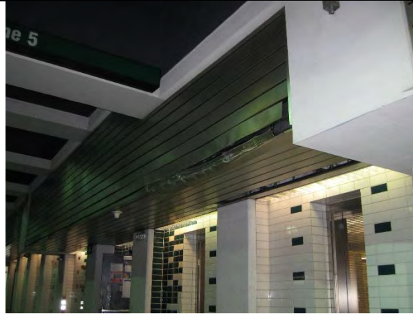
Damaged fascia in bus tunnel
