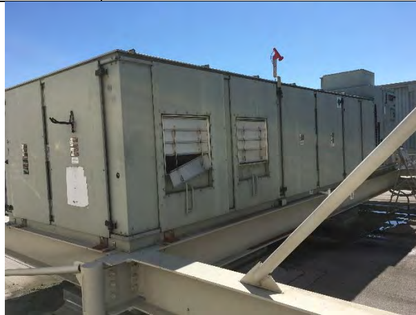
Two largest HVAC units on the roof
