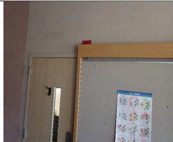
Fire alarm horn is obstructed by display in Alder Conference Room
