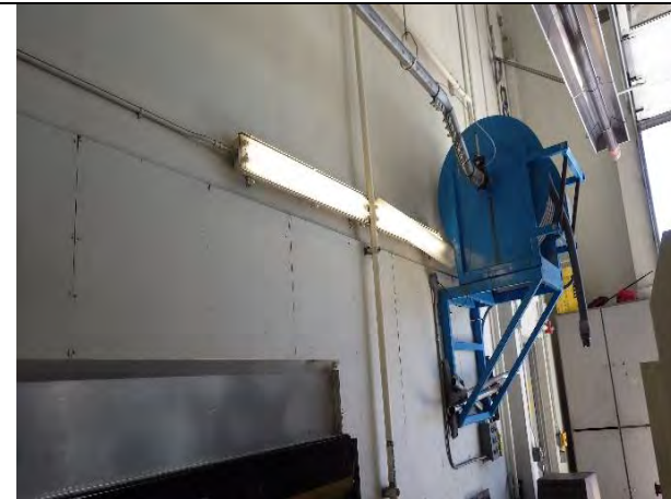
Lights in quick check service bay
