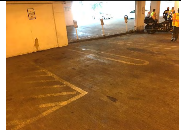
Parking lot striping has faded and needs repainting
