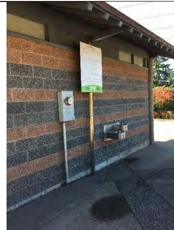
Utility meter and water fountain on utility building
