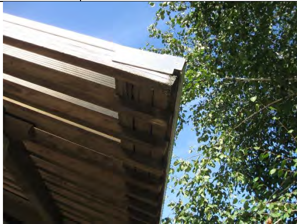
Bus shelter gable end roof rafters rotted
