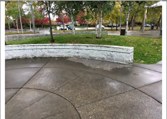
CMU seating needs paint
