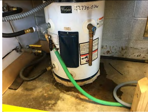
Hot water tank in utility room
