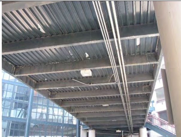
Peeling paint on underside of pedestrian bridge
