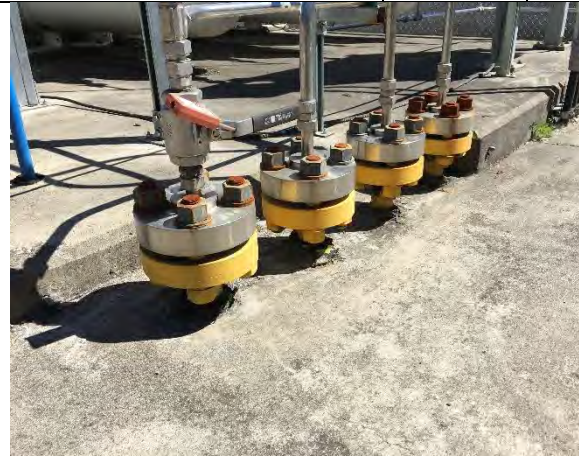
Rusty bolts on compressed natural gas flanges
