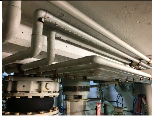
Condensation collecting on the small piping near the chlorine injection system
