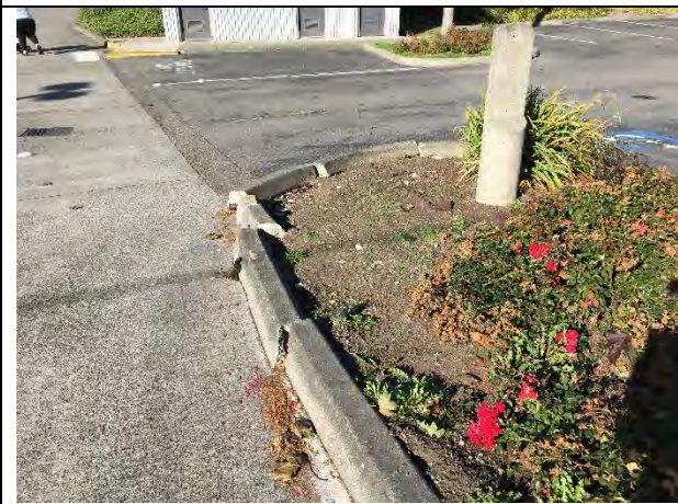
Broken curb just south of utility building
