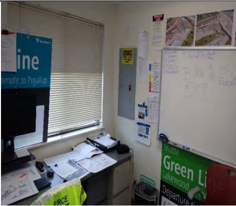
Electrical panel in service supervisor office
