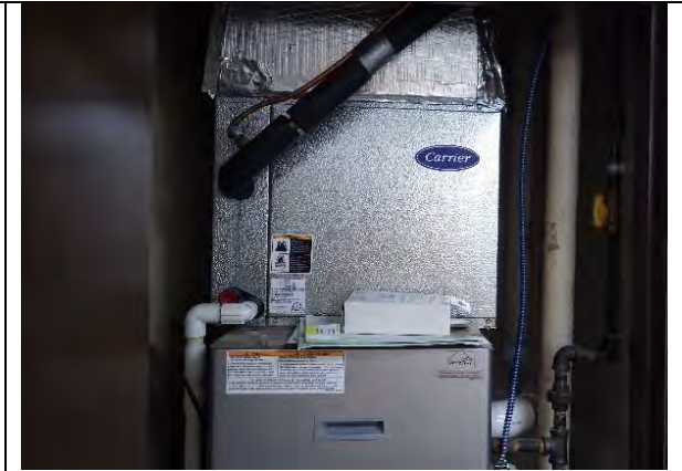
MC cable in need of support
