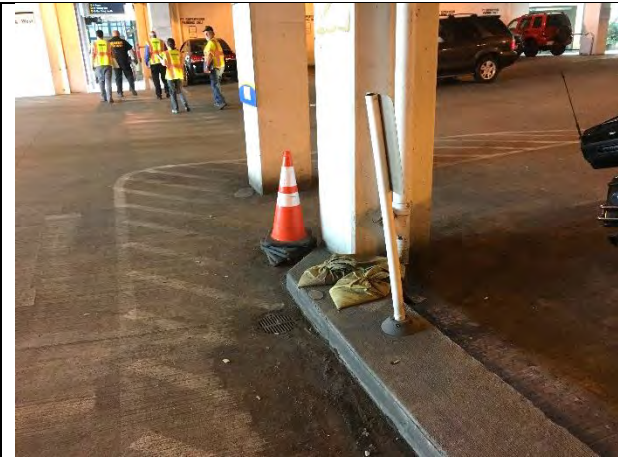
Parking lot striping has faded and needs repainting
