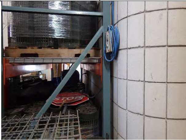
Overhead lighting in tent storage fed by extension cord
