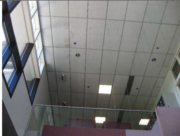
Water stains at high ceiling over main entry
