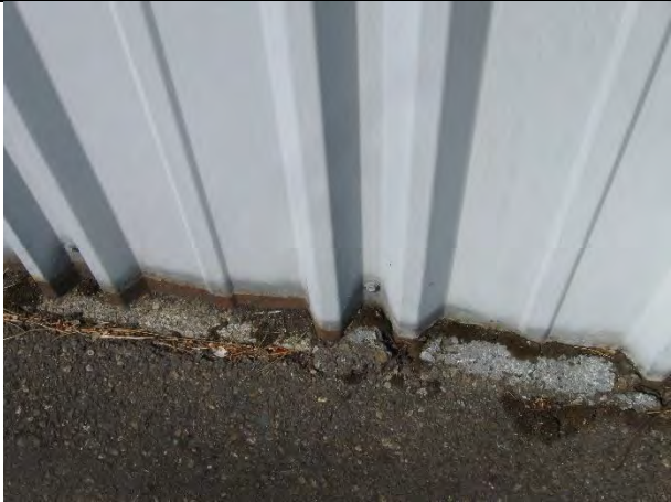
Asphalt covering bottom of metal siding
