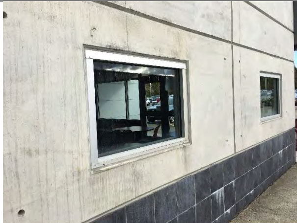
West wall of building, showing lunchroom windows and stains at wall tile joints
