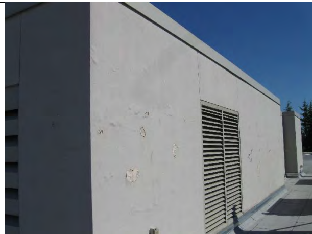
Peeling paint on south side of penhouse
