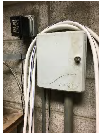
Irrigation system in utility room
