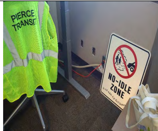
Executive Office cubicle work station missing electrical cover plates
