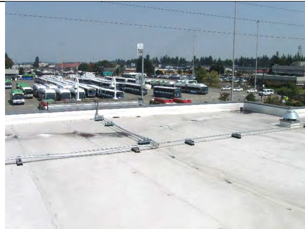
View of roof looking north, showing some low spots with debris and roof mounted conduit runs
