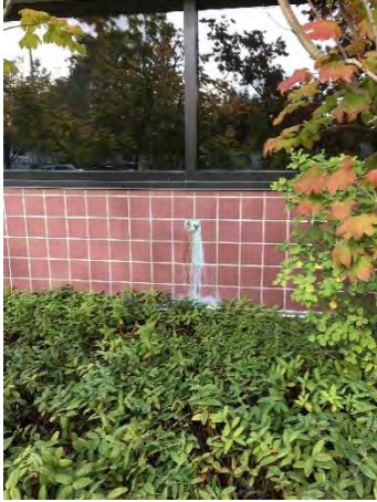
A hose bib on the front of the building appears to have a very slow leak and has caused a scale buildup down the side of the building
