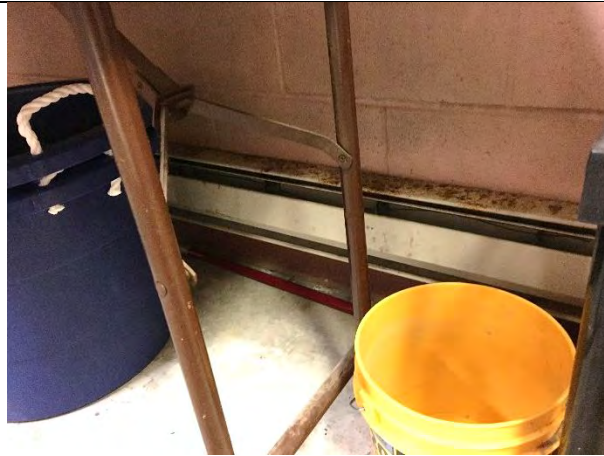
Baseboard heater along north wall has items stored too close
