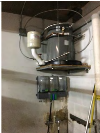
Water heater in storage room with mop sink
