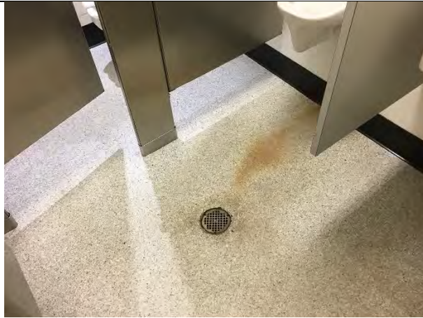
Staining on floor in front of urinal
