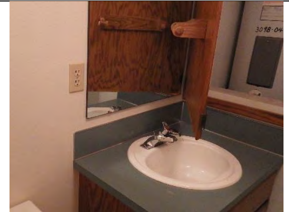
Replace receptacles with GFCI protection
