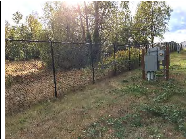
Modular Office electrical service
