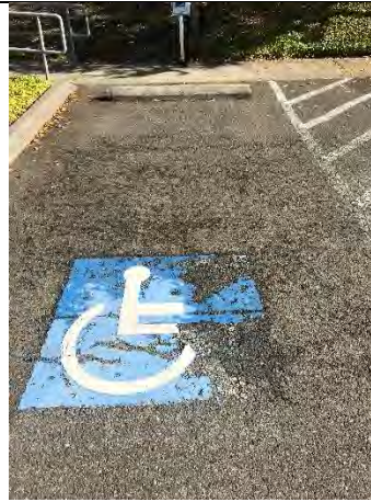
ADA stall asphalt paint needs repainting
