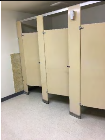
Women's restroom partition walls
