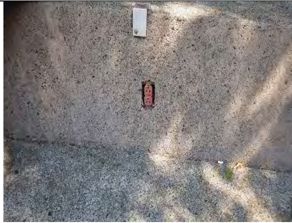
Receptacle in south end of upper plaza missing weatherproof cover
