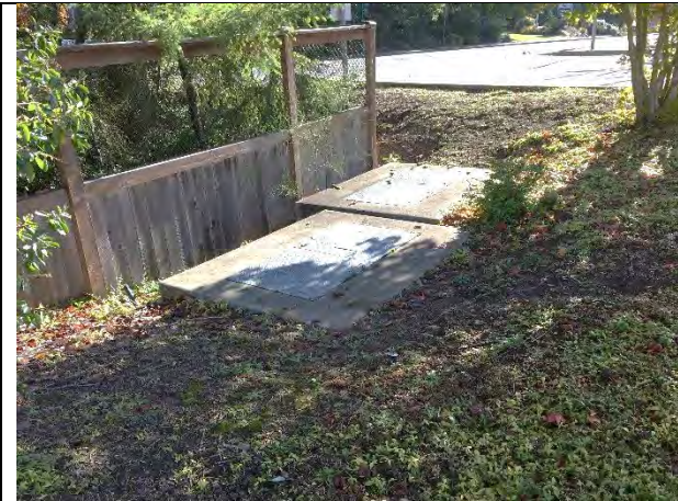
Site service vaults
