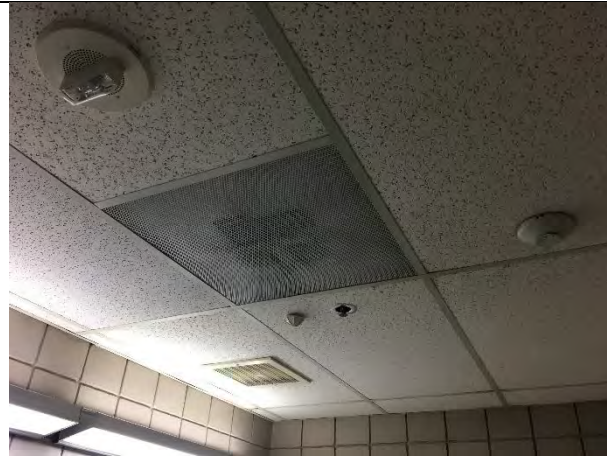
Exhaust fan in restroom functional
