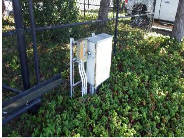
Non-functional gate opener on north side of employee parking lot
