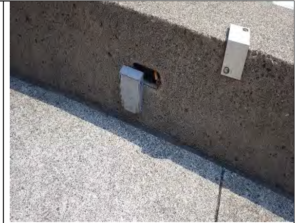
Junction box at north end of plaza have receptacle missing leaving access to exposed conductors
