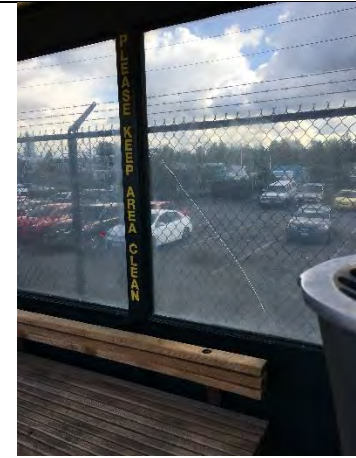
Smoking shelter window is cracked
