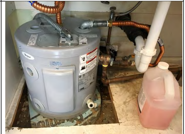
Water heater tank in the staff room near the public restrooms
