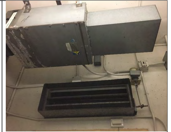
Pump Room fan in Electrical Room
