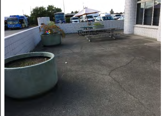
Cracked concrete slab on patio, outside lunch room
