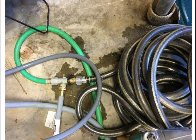
Hose bib connection in utility room
