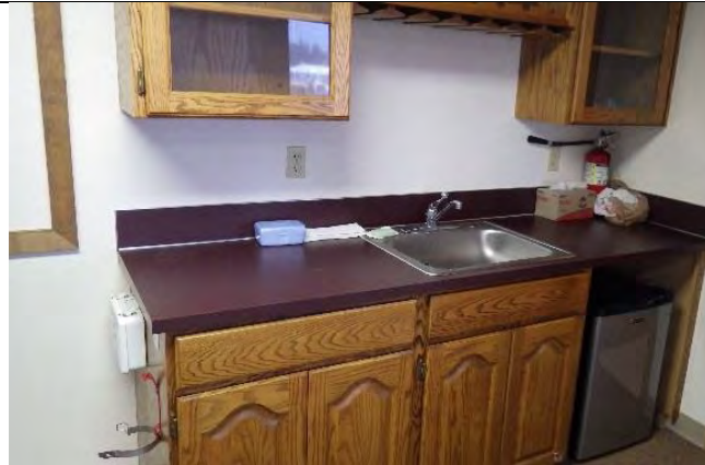
Replace receptacles with GFCI protection
