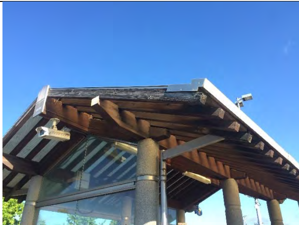
Bus shelter gutters and downspouts
