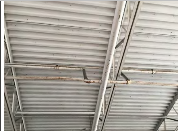
Rusted exterior dry system piping
