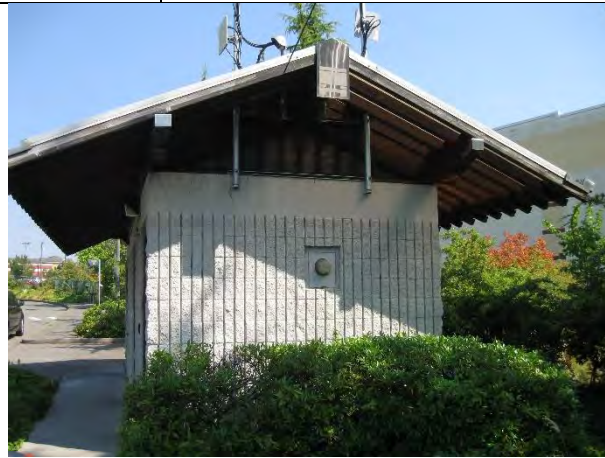
Power meter on utility building
