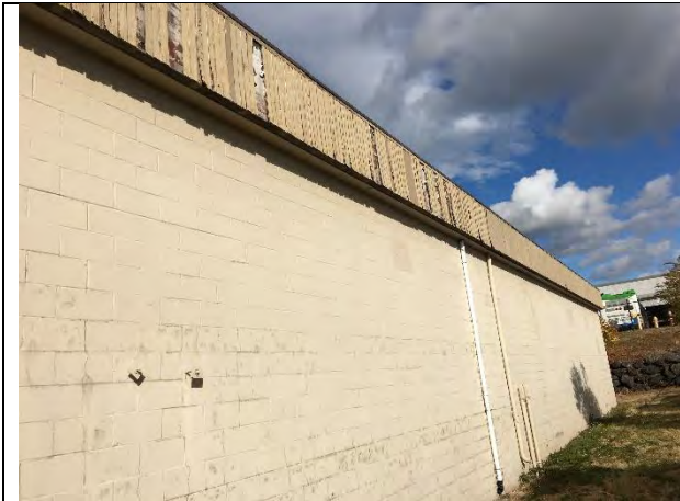
Damaged façade trim
