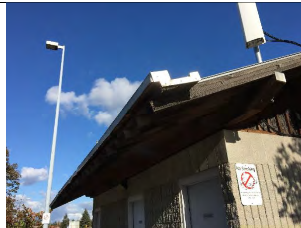
Utility building showing gutters with no downspouts
