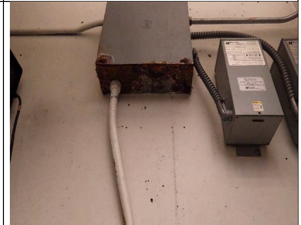
Junction box in main electrical room has severe corrosion and should be replaced
