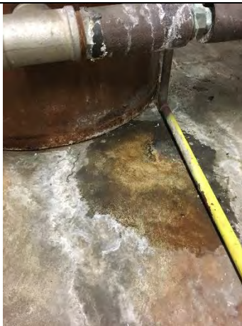
Slow leak near the larger water heater in the mechanical room
