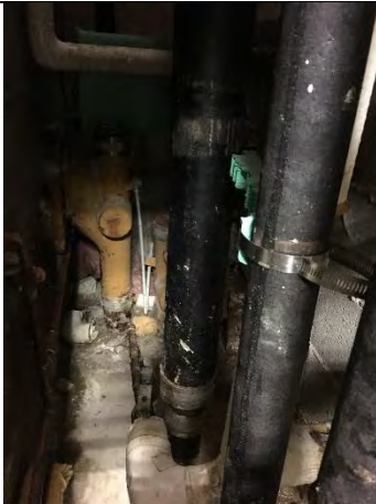
Difficult access for maintenance and repair for the water distribution and sanitary waste for driver break room/rest area
