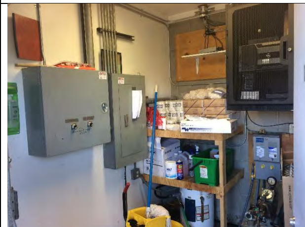
Utility room in utility building
