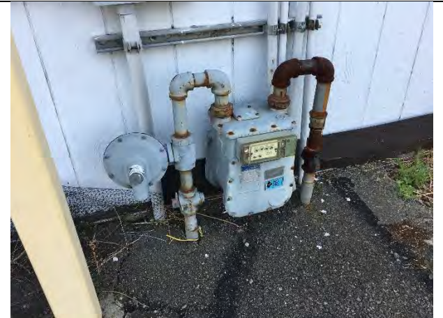
Gas meter and appurtenances
