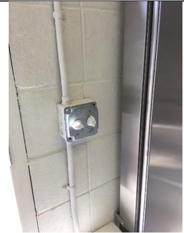
Restroom exhaust fan and light timers
