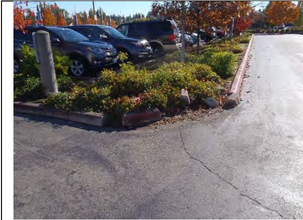
Broken section of curbing
