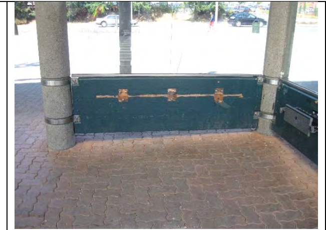
Missing seat in south bus shelter
