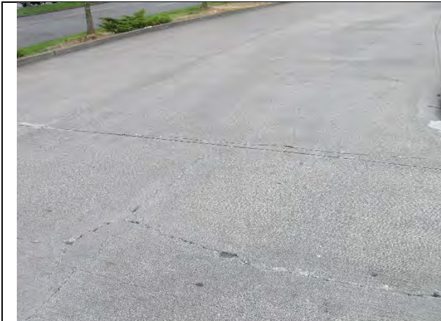
Cracks along interior roadway
