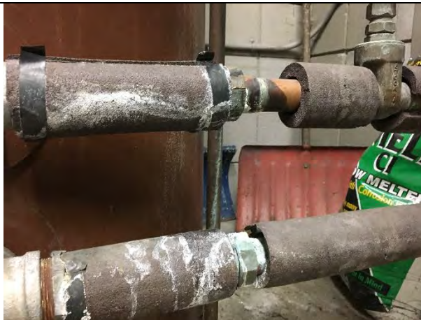
Slow leak near the larger water heater in the mechanical room
