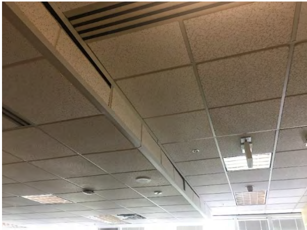
Sprinkler heads near soffit
