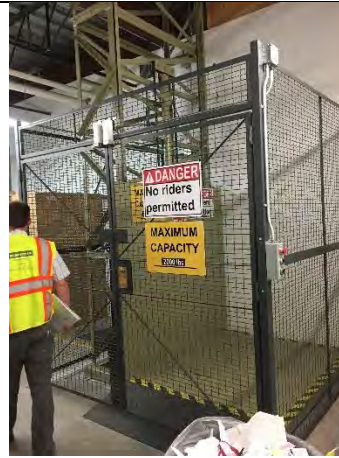
Maintenance lift first floor
