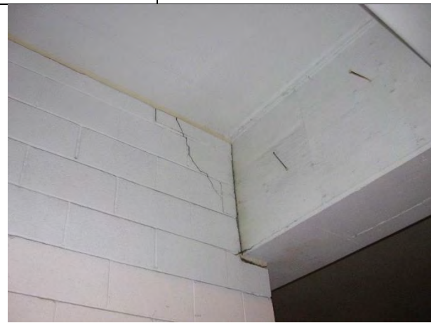
East garage- broken CMU in northwest corner
