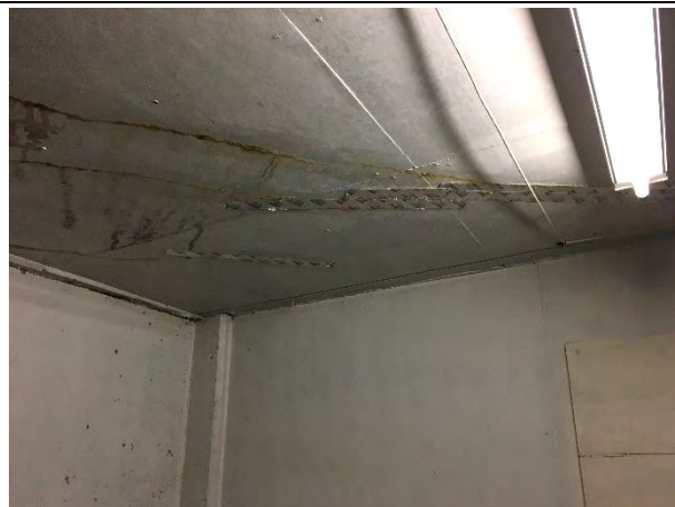
Electrical/controls room in the west parking garage, cracks/leaks in ceiling repaired with sealant tape
