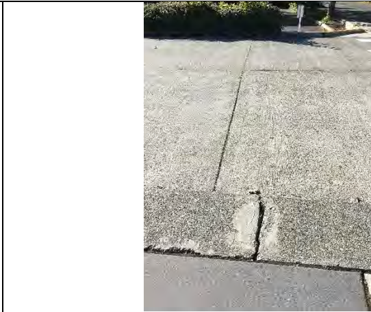
Cracks in sidewalk need repair
