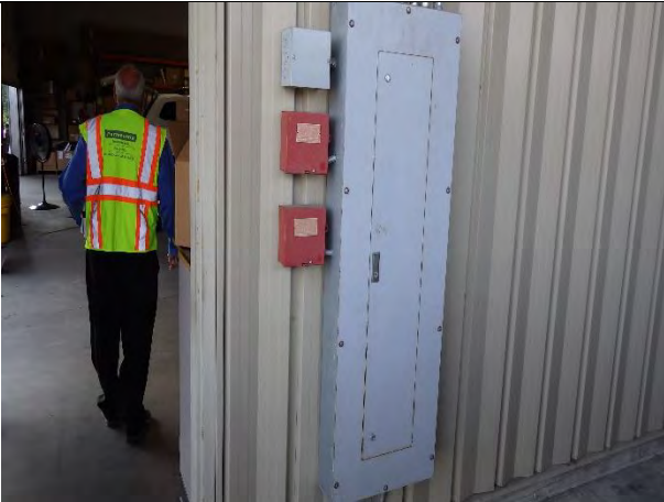
Restore protective coating on panel enclosure
