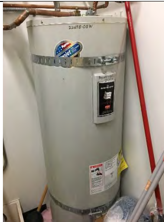
Water heater in utility room
