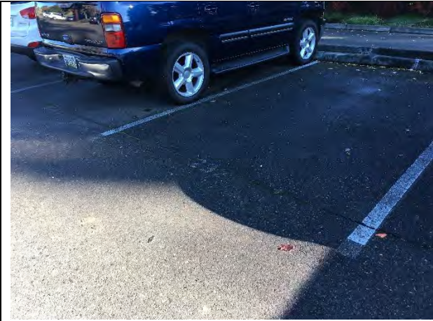
Parking striping and numbers in need of repainting
