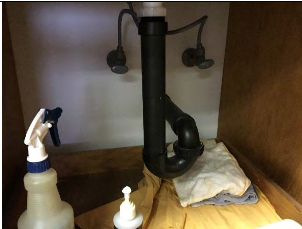
Office/locker building under sink on second floor
