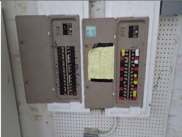
Electrical service in working order
