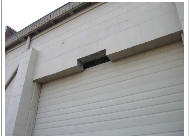
Door header cut out at north door on west wall
