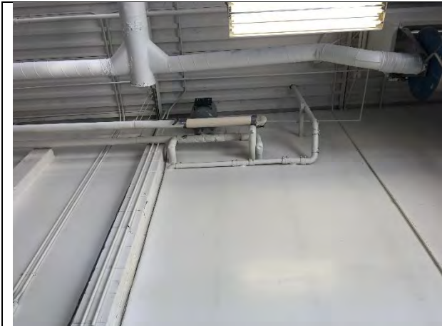
Evidence of repaired water distribution piping from small leaks
