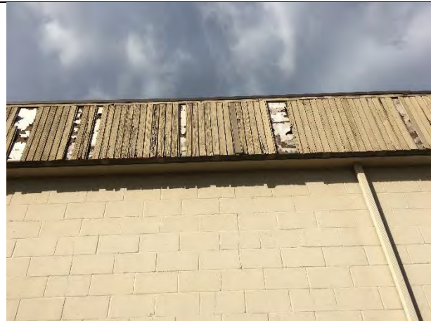
Damaged façade trim
