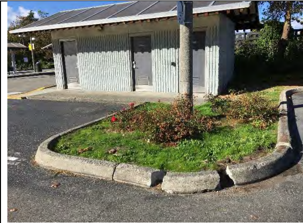
Broken curbing in front of Utility Building
