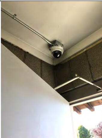
Cameras installed inside utility room and around site
