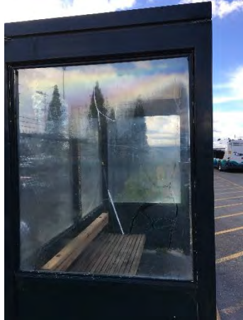
Smoking shelter window tint is splitting
