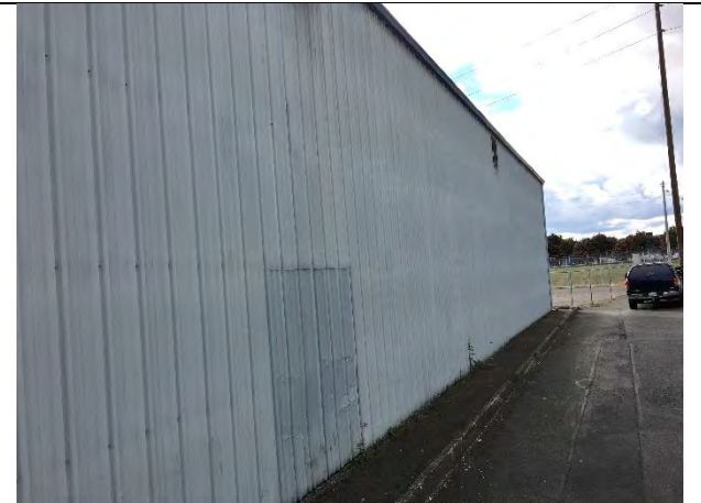
Patched siding on north wall of building
