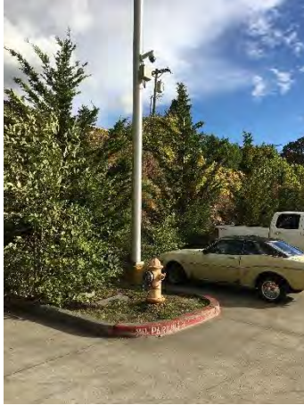
Fire hydrant on east side of parking lot
