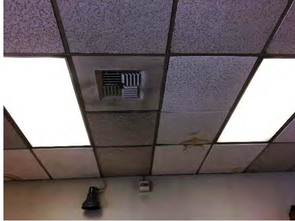
Water leak stains on north wall of fare counting room
