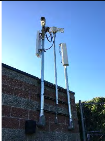
Cameras and radio communication located on utility building
