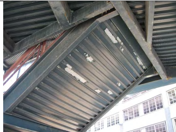
Peeling paint on underside of stairway
