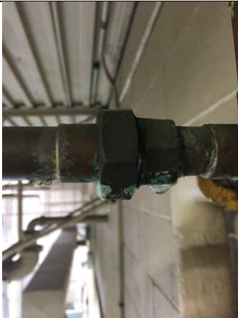
Close up view of cold water piping leak
