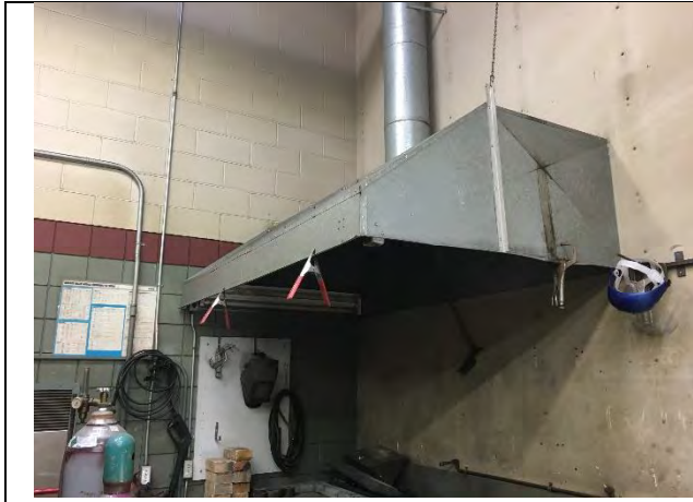
Functioning exhaust hood in shop
