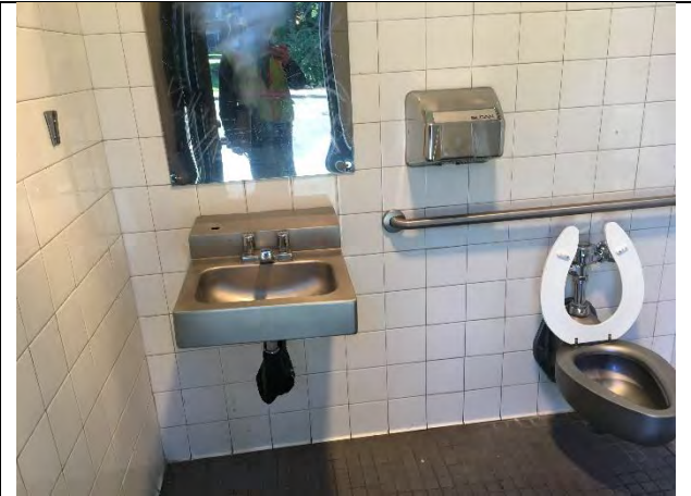
Sink and toilet in public restroom
