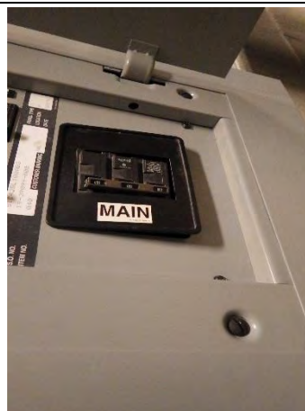
Plastic trim around the main breaker in Panel P1 (East Garage Electrical Room) is not seated properly
