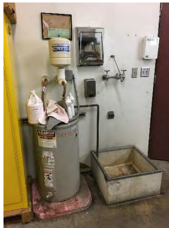
Water heater tank in the facilities maintenance work room
