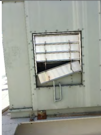
Roof mounted HVAC units gravity damper blade
