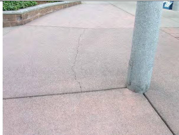
Cracks in concrete walkways
