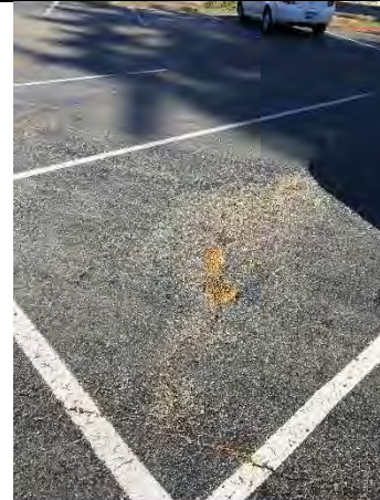
Alligatored asphalt in parking lot with plant growth in cracks
