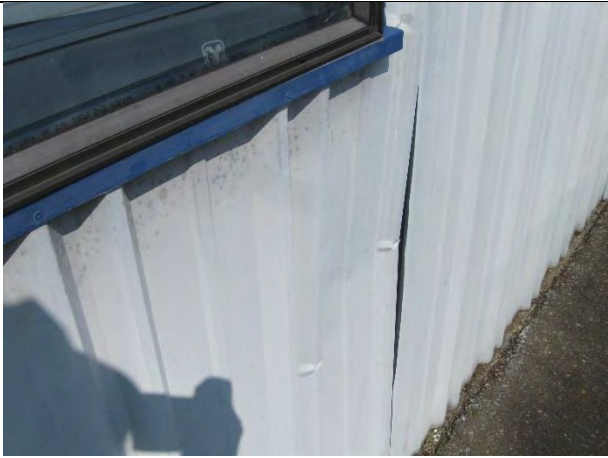
Dents in metal siding at east wall
