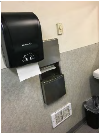
Wall heater in men's restroom
