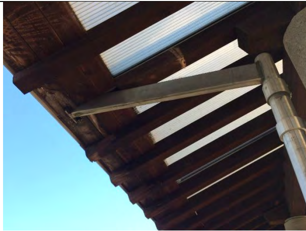
West bus shelter showing rot at downspouts
