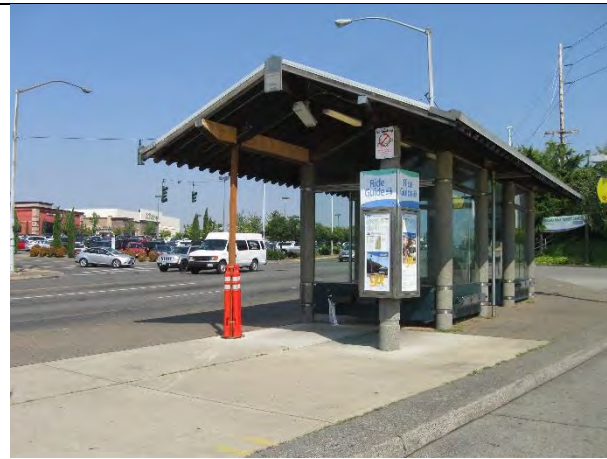
North bus shelter with wood post shoring roof beam
