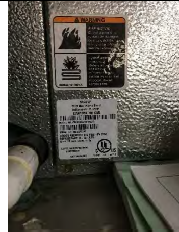
Interior of HVAC system for service supervisors building
