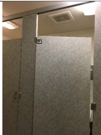
Exhaust fan in men's restroom
