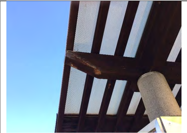
West bus shelter rot damage
