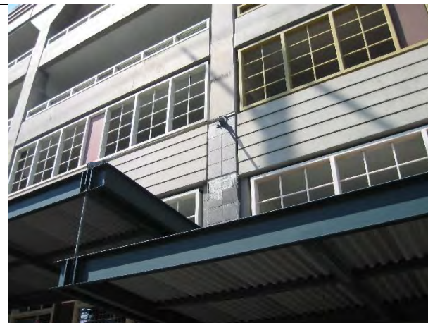
Missing tile approximately 20 feet west on south wall of east garage
