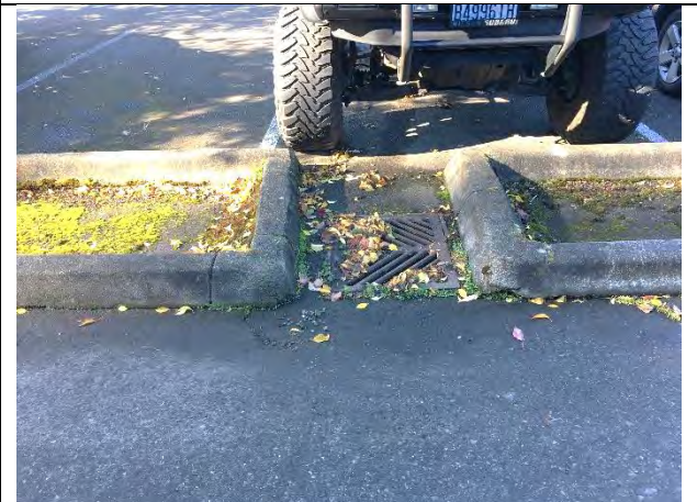
Storm grating in parking area
