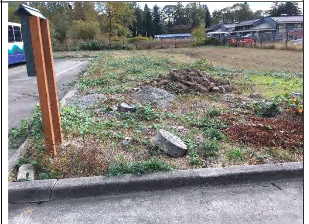
Landscaping in southwest corner of parking lot
