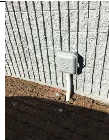
Communication box on outside of utility building
