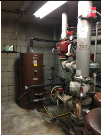
Hot water tank has exceeded expected typical lifespan
