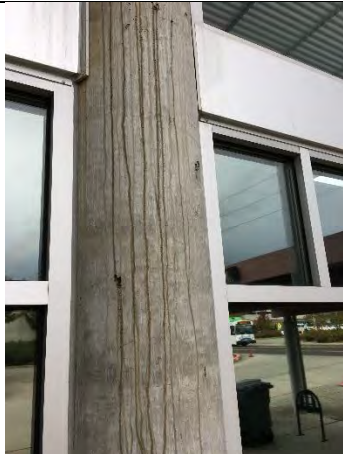
Voids and streaks on concrete columns at northeast side of entry
