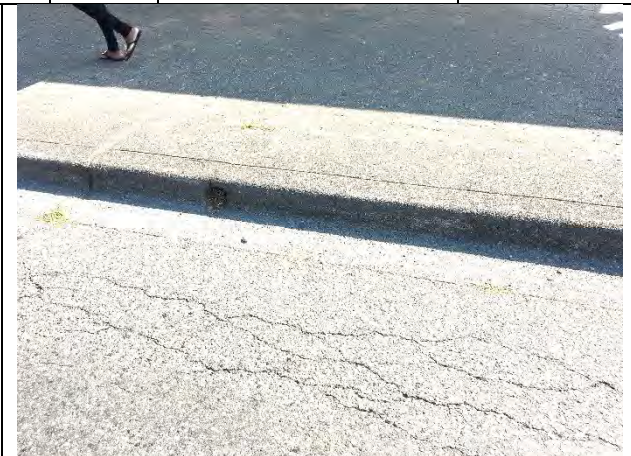
Shelter drain appears to be clogged
