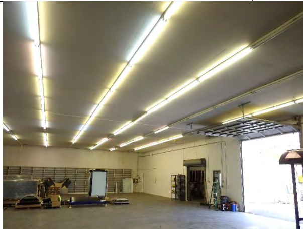
Lighting in main bus shelter work area
