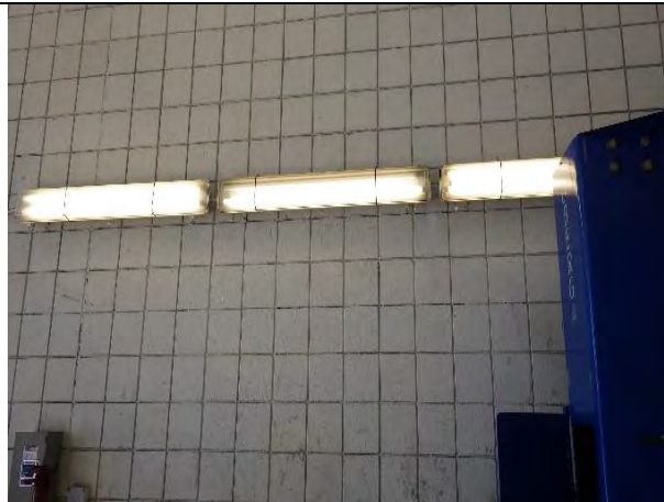
Lights in quick check service bay
