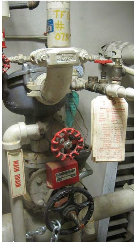
Fire Riser (Dry System Valving)
