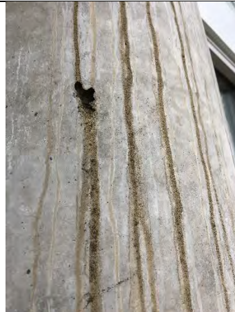
Voids and streaks in concrete columns at northeast side of entry
