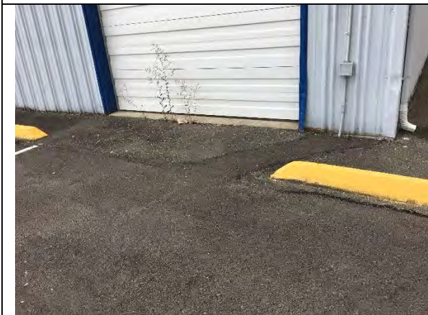
Weeds in the cracks between the asphalt and foundation
