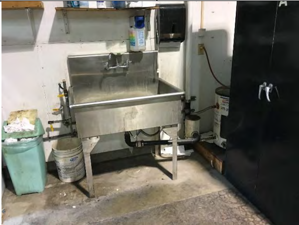
Sink in radio maintenance area
