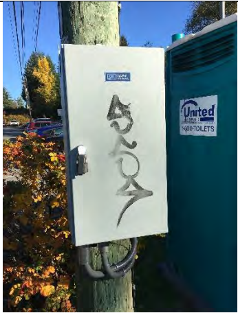
Control cabinet with graffiti
