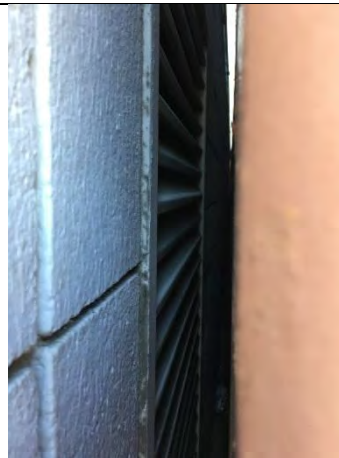
Exterior wall louver for mechanical/electrical room covered by shipping container directly next to building
