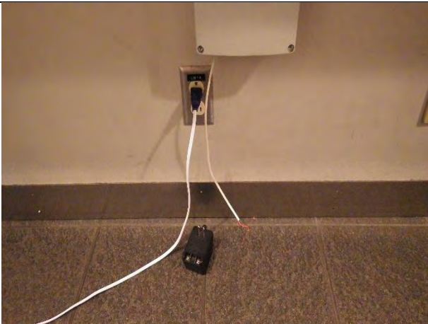
Unknown piece of low-voltage equipment located on wall under counter in the Operator's lobby has disconnected plug in transformer
