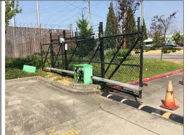
West vehicular gate not in working order
