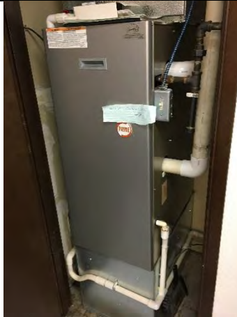
Interior of HVAC system for service supervisors building
