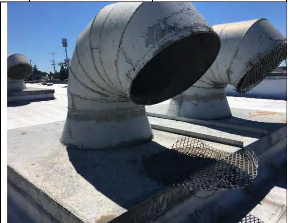
Screen for fuel island exhaust vent has fallen off
