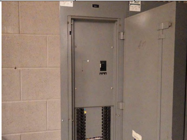
Electrical panel A7 on the first floor
