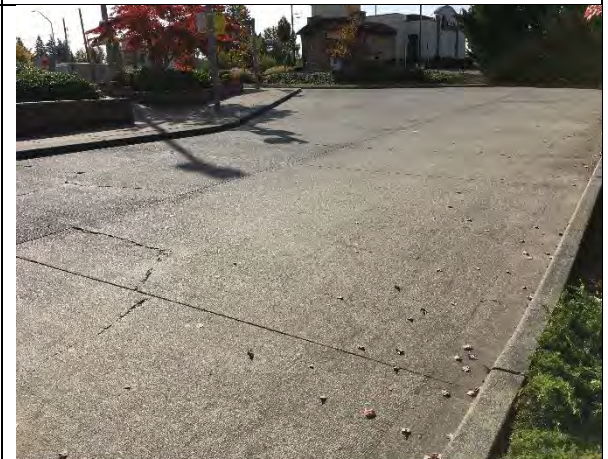
Cracks in interior roadway concrete
