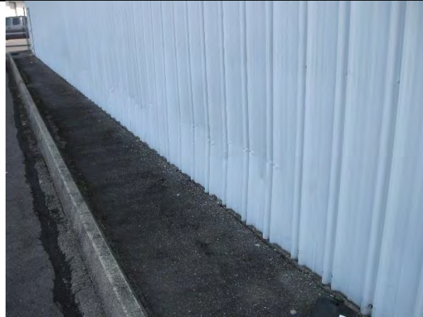
Asphalt fill and dented siding along west wall
