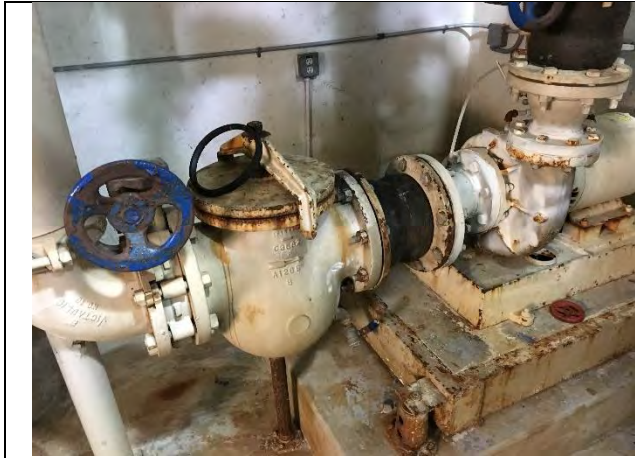
Pump room – corrosion throughout
