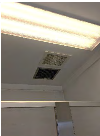
Restroom fluorescent tube lighting
