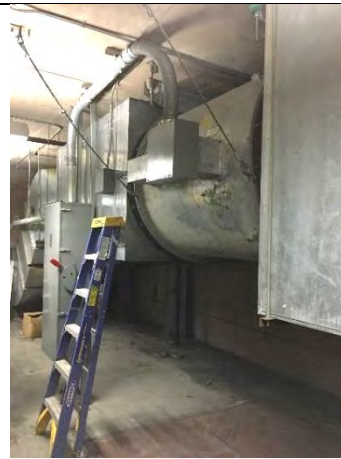
Large fan above bus tunnel entrance
