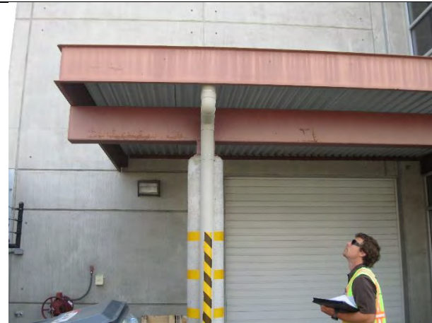
Steel beams at loading dock, northwest corner. Beams have some rust appearing
