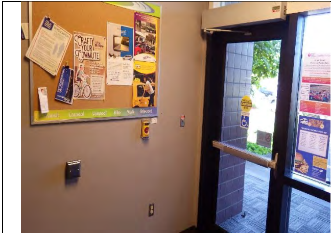
Single exterior door on north side of building with ADA opener does not function properly
