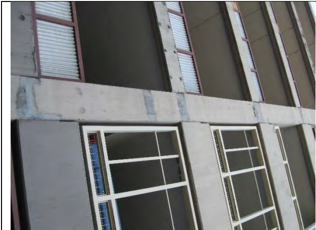
Column to beam joints on east garage showing patched cracking
