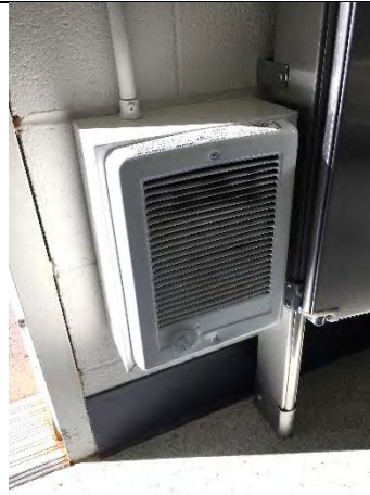
Women's restroom unit heater
