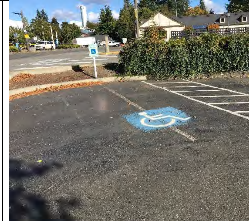
Disabled parking stall needs repainted
