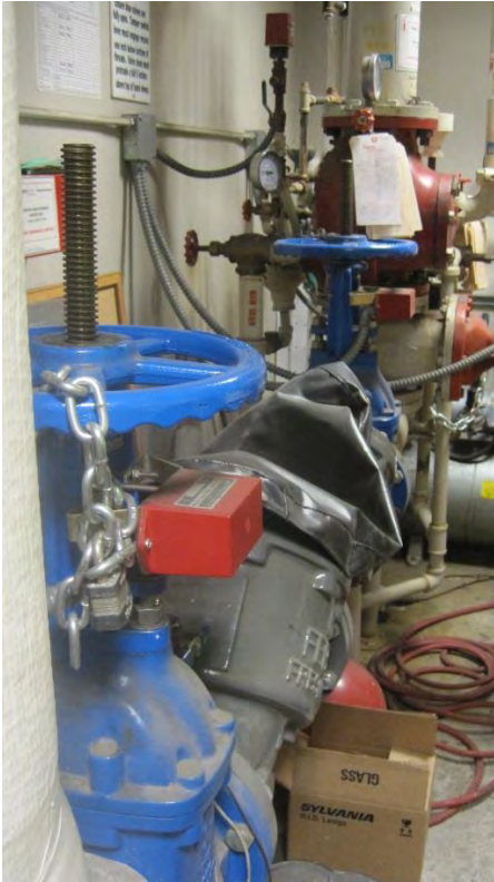
Fire Riser (Dry System Valving)
