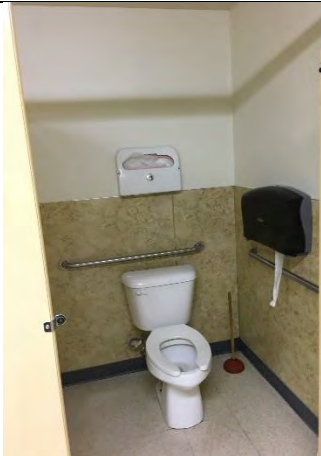
Women's ADA stall does not meet ADA requirements
