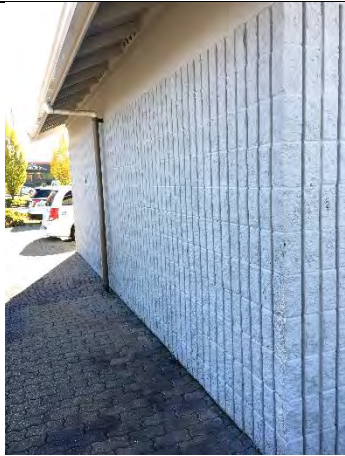
Utility building downspout
