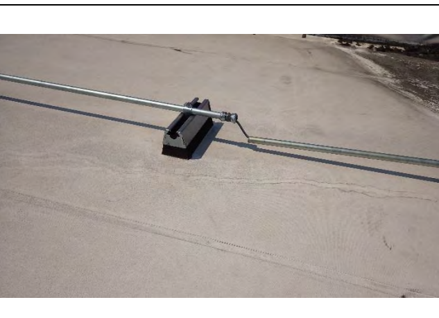
Conduit separated on roof to be repaired
