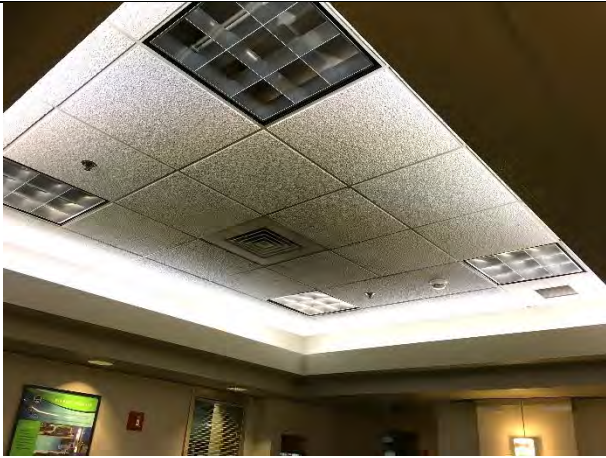
The driver break-room/rest area cooling system
