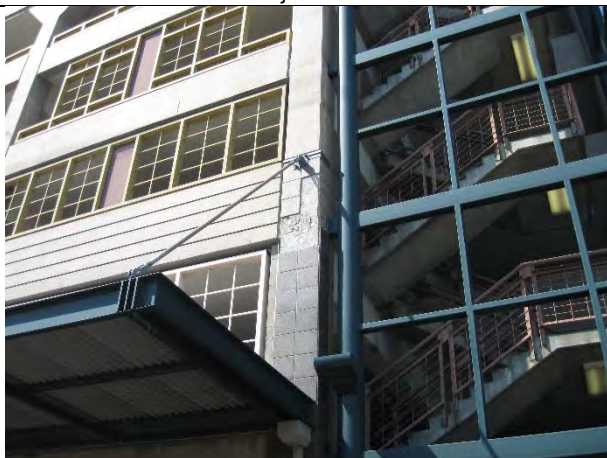
Southeast corner of east garage – missing tile under canopy support rod
