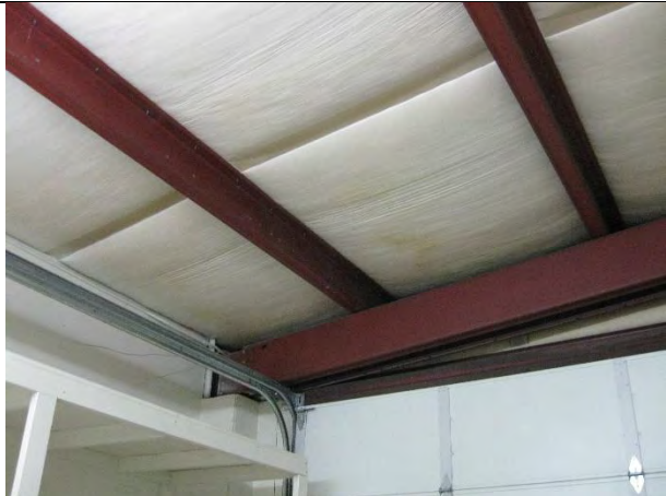
View of roof framing and insulation above roll-up door in shipping room
