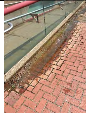
Water was collecting at the top of the wheelchair ramp near Broadway
