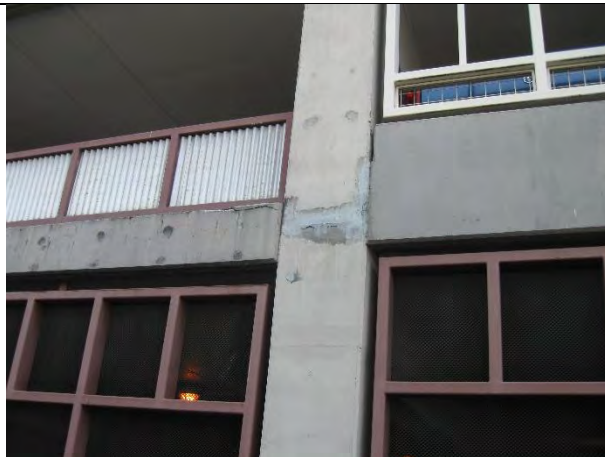
Column to beam joints on north wall of west garage showing patched cracking
