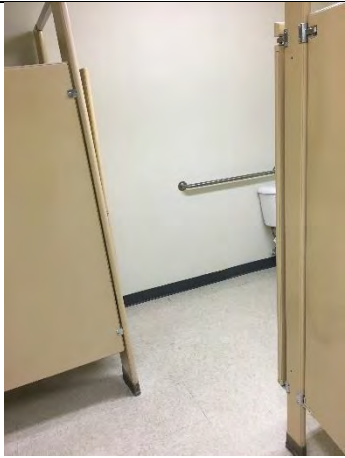
Stall defined as ADA, but does not meet ADA design requirements
