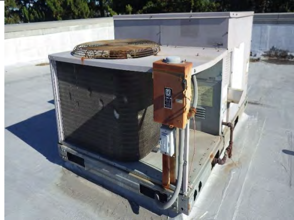
Roof mounted unit is aging and shows signs of surface rust
