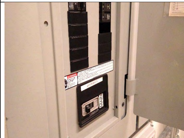
Panel R5 Breaker
