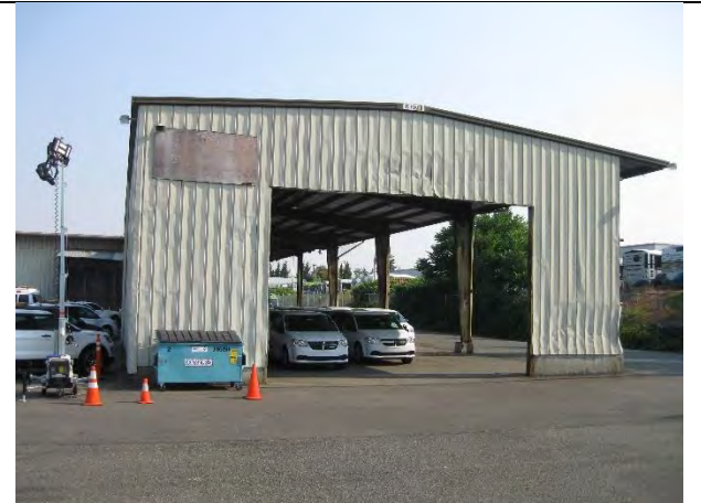
South wall of "L", showing damaged siding
