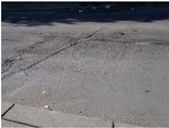
Asphalt near concrete paving needs repair
