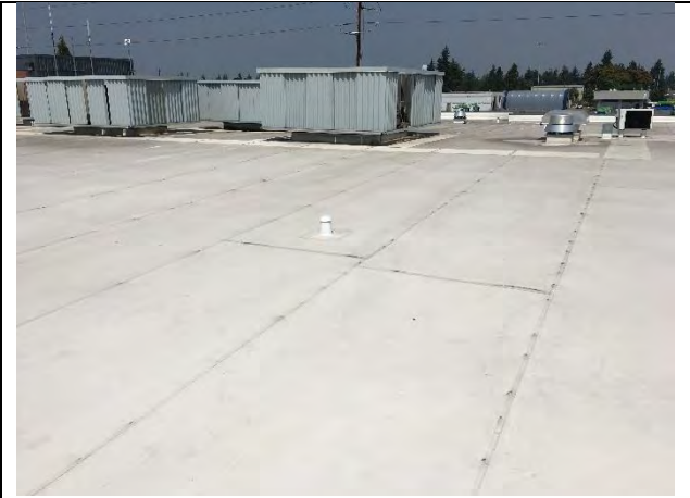
Roof, showing screening at roof mounted HVAC equipment
