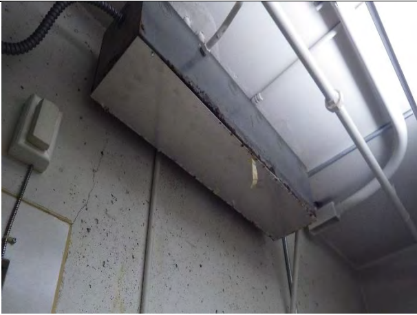
Electrical gutter in storage room has severe corrosion and should be replaced
