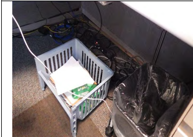
Executive Office cubicle work stations located in old second floor lobby area currently have power strips plugged into power strips or other means of temporarily adding receptacles
