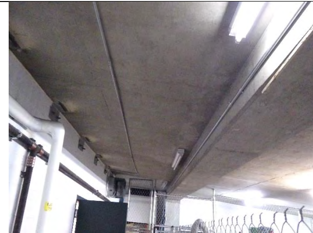
Two fluorescent lights were not functioning and the third in photo was pulsating
