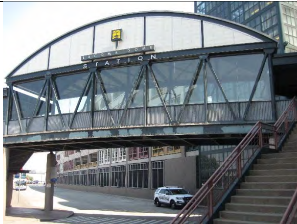
Steel structures at north side shows paint peeling and rust at joints
