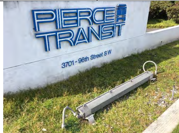
The bracket for positioning the lighting on the east side of the large, street facing Pierce Transit sign is broken
