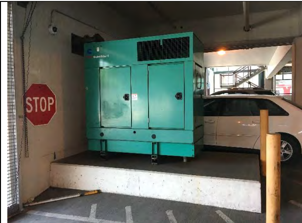
Generator in East Garage
