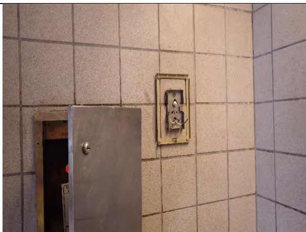
Thermostats have been removed
