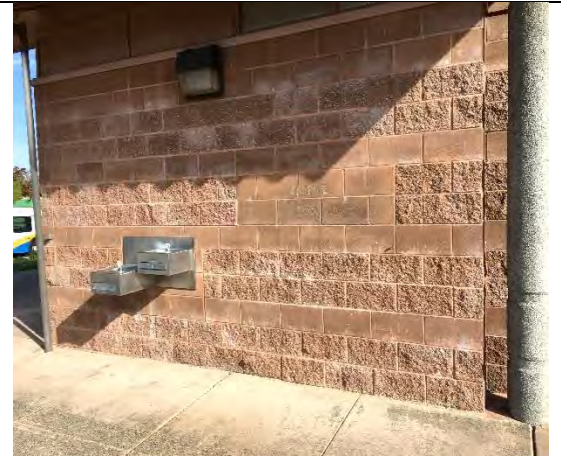
CMU walls need cleaning
