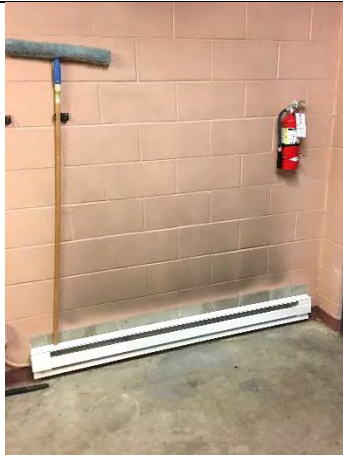
Baseboard heater in utility room
