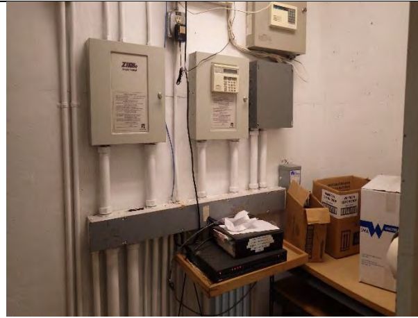
Signs of water dripping on security equipment
