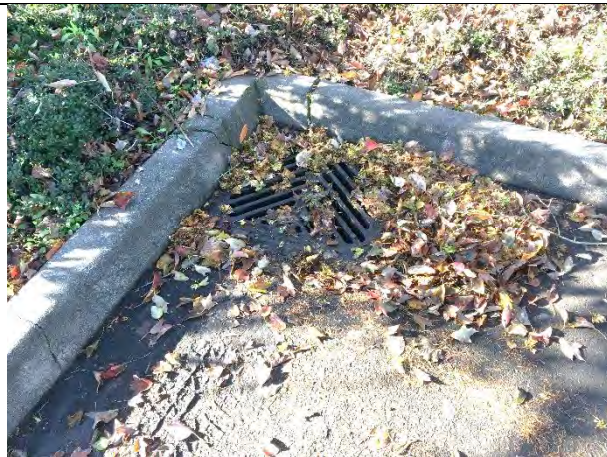
Storm grate covered by leaves (leaves were moved for photo)
