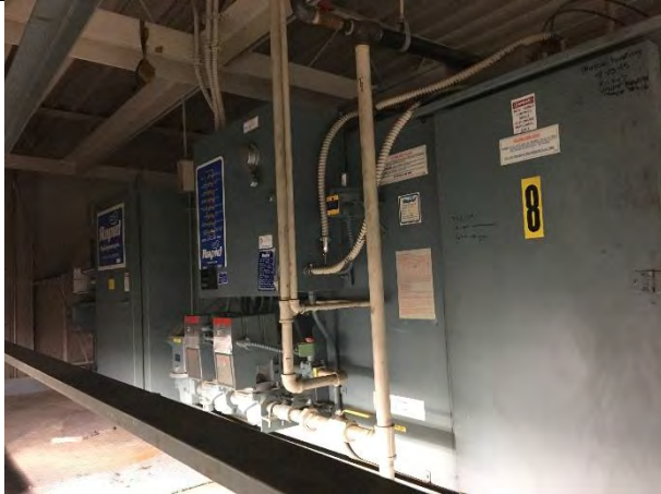
Heating and cooling systems provided for building is natural gas
