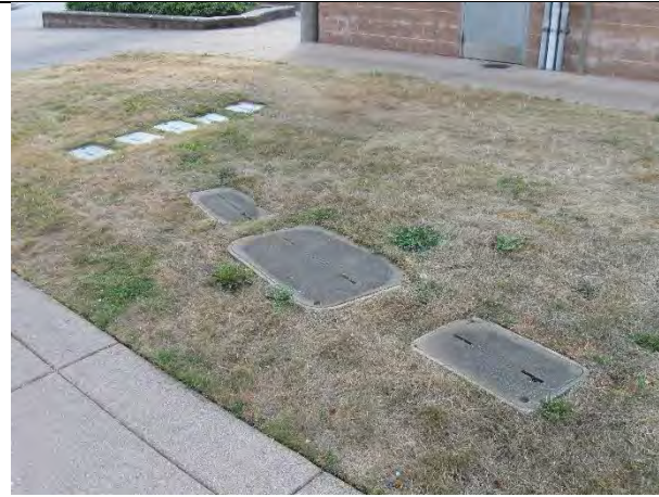
Telephone, electric, communication, and irrigation vaults
