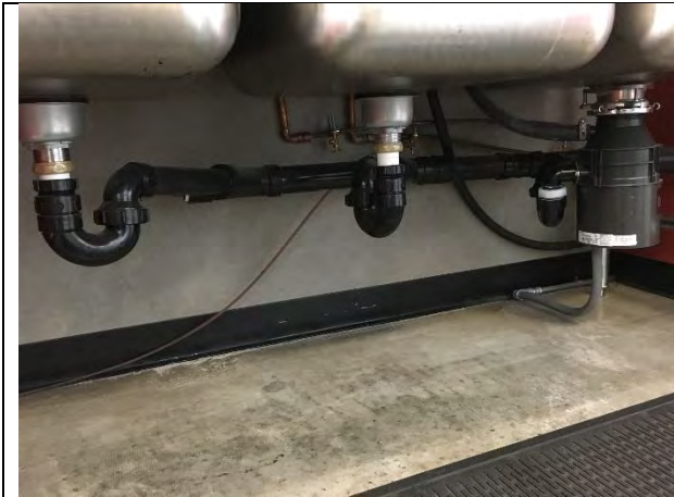
Plumbing under kitchen sink in good working condition
