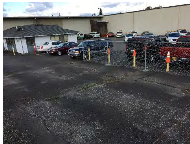
Cracks in asphalt where grass and weeds are growing through
