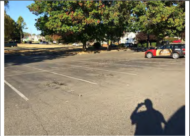
Parking lot striping and numbers are fading
