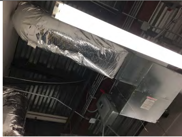
HVAC ducts in storage room
