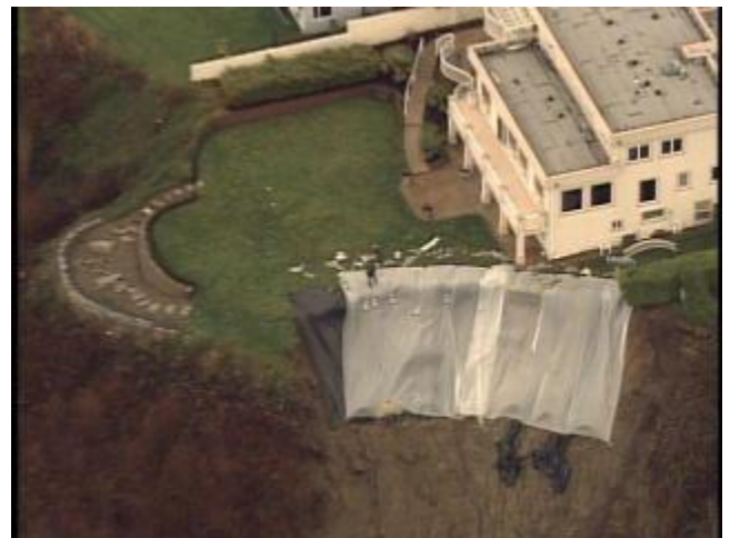
Figure 4.3-1 Northeast Tacoma – Landslide 01/2007
