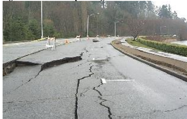
Figure 4.2-5 Lateral Spreading –March 2001
