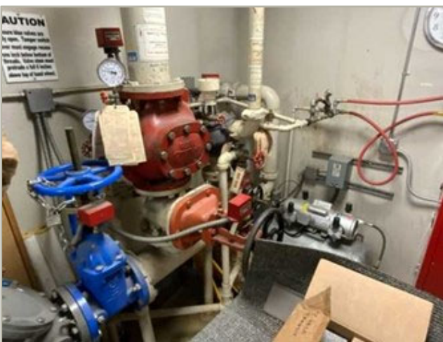
5 - FIRE SYSTEM PIPING
