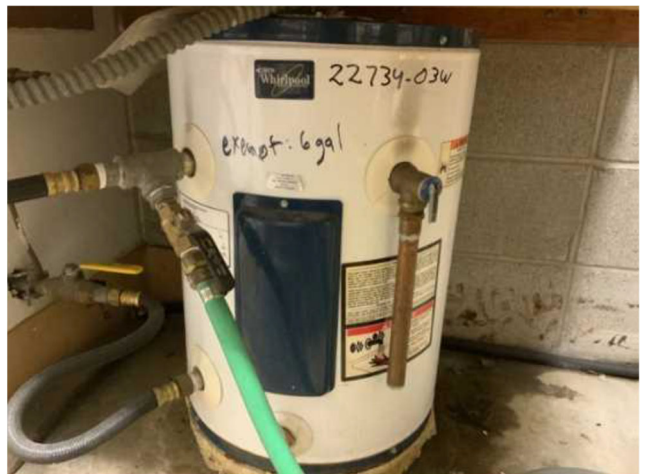
4 – ELECTRIC WATER HEATER
