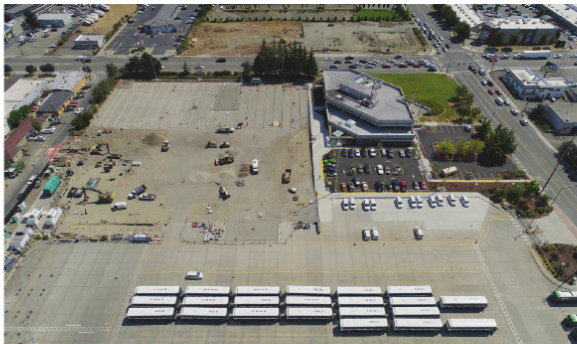
An aerial view of the Pierce Transit MOBI project featuring parking improvements west of Building 4 and site preparation for the new fuel and wash building north of Building 4.
