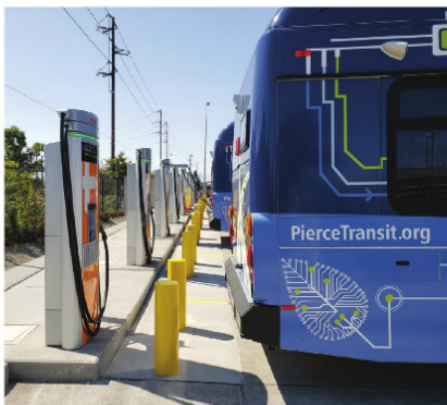
A key element of the new MOBI facility, here are Pierce Transit electric buses parked and charging.
