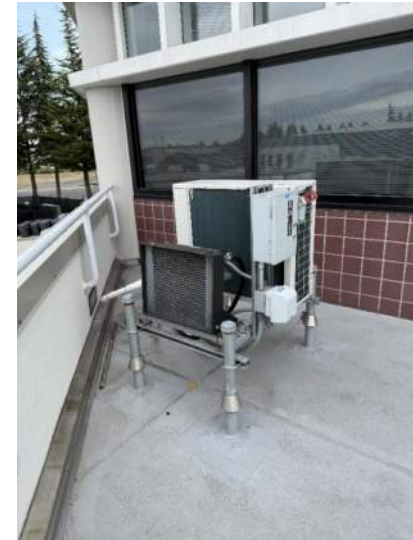
Exterior cooling units for elevator mechanical room.
