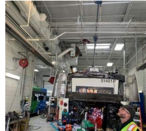
Overhead fall protection equipment for on-top-of-bus work.
