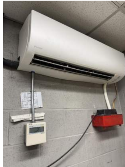
Interior air handler unit for cooling elevator mechanical room.
