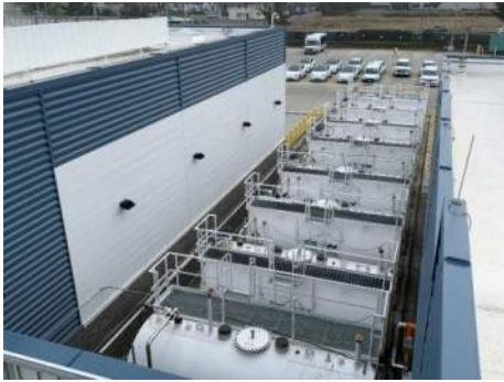
Fuel Tanks, viewed from roof
