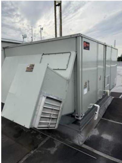
Rooftop HVAC unit with vibration that should be repaired.
