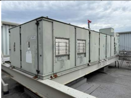
Large rooftop mounted HVAC unit.
