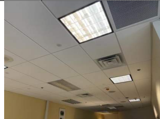
HVAC supply and return vents in ceiling.
